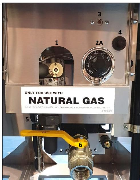
Control Panel A
