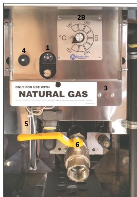
Control Panel B
